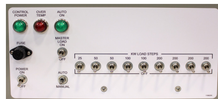
Remote Manual Control Panel shown.
