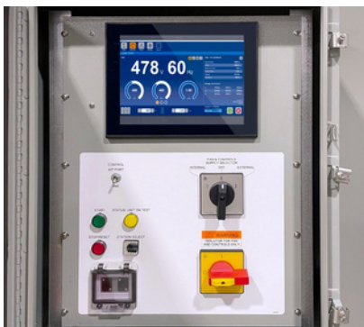
Control Enclosure with SIGMA 2 interface panel and HMI screen.
